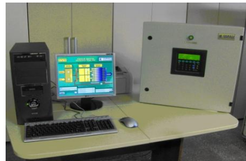
Wastewater Treatment Plant Monitoring and Control
